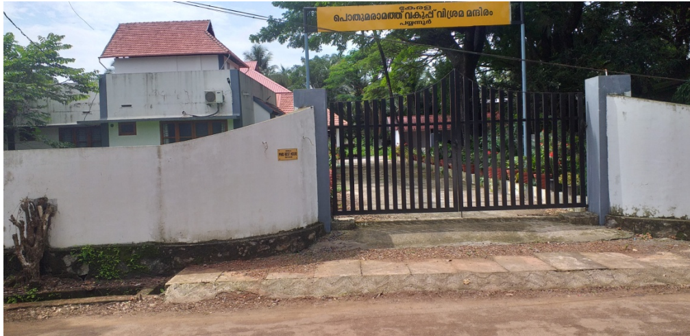
affected PWD Rest house wall and gate
