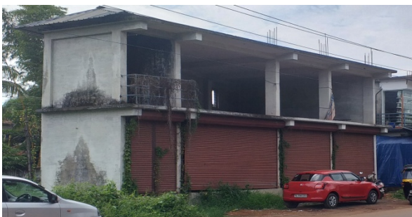
Commercial building affected
